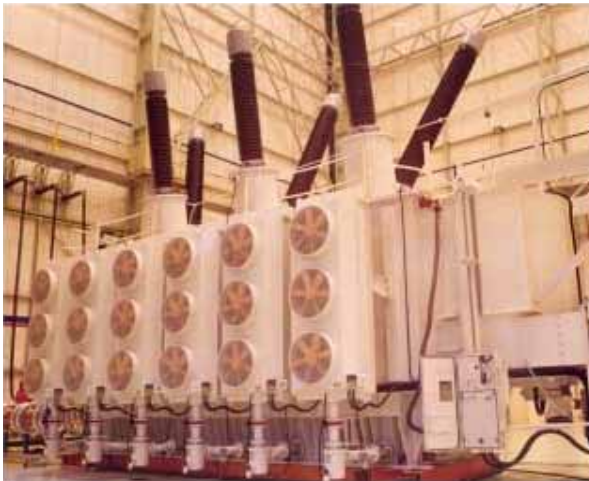
450 MVA auto-connected system intertie transformer
