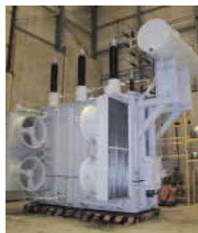
64 MVA Drives Converter Transformer. 12 pulse
