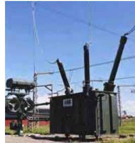
Shunt reactor, 400 kV, 150 MVAR
