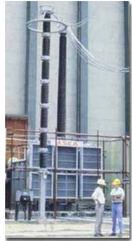
Oil-immersed smoothing reactor in the Rihand - Dehli HVDC transmission
